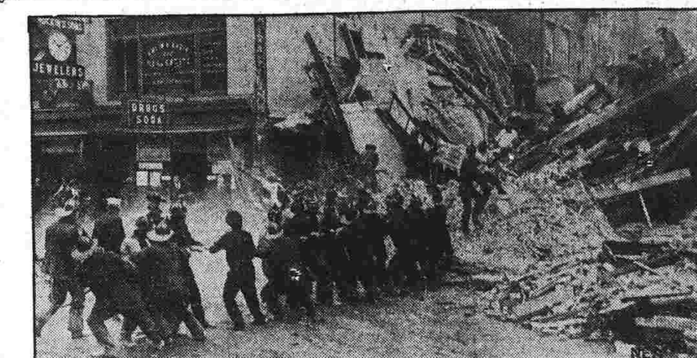
It was a grim tug-of-war with death that these New York firemen staged when a building undergoing repairs collapsed, pinning workmen beneath the debris. Here you see a steel girder being pulled off the wreckage to speed the search for victims of the cave-in. More than ten persons, including passers-by, were injured; several were missing.
